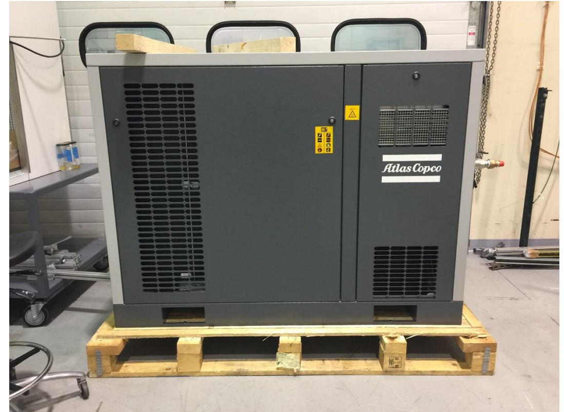
Air compressor for cooling system in EEL 125.
